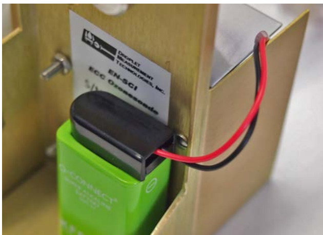
Figure 34 Battery Wires Running Between the Ozone Sensor Frame Wall and the Ozone Sensor
